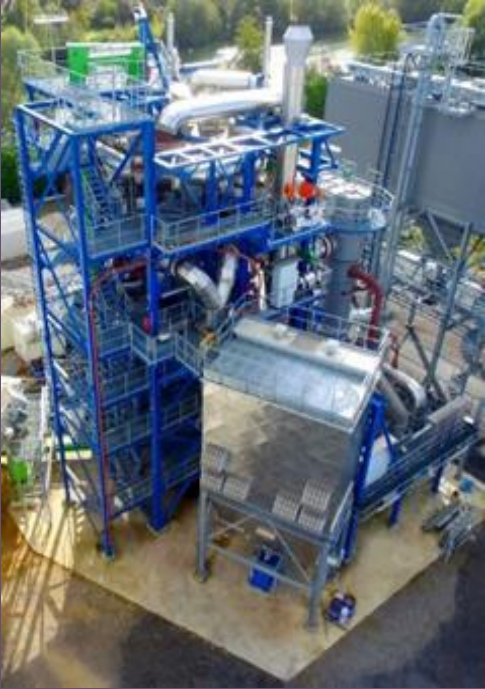
Drying + Torrefaction Venette, France Capacity: 3 t/h biomass
